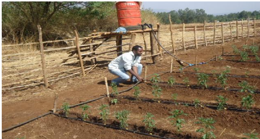
Figure 2: Installation of family drip irrigation for verification on pawe agricultural research center station.
